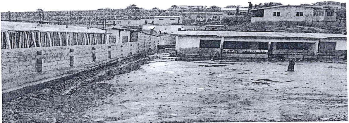
Illegal construction of houses in waterways
