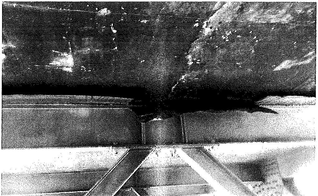
Figure 14. Yapei Bridge. Space between diaphragm top cross beam and concrete deck.
