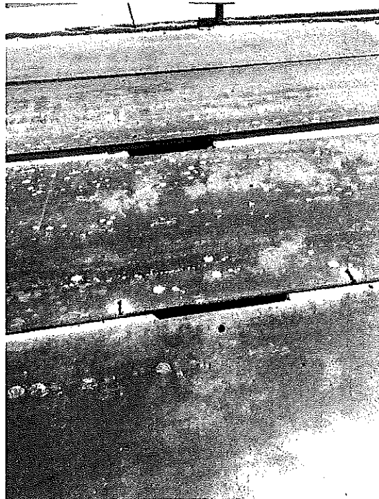
Figure 26. Yapei Bridge. Steel plates spanning the void in the concrete deck in an intermediate joint.
