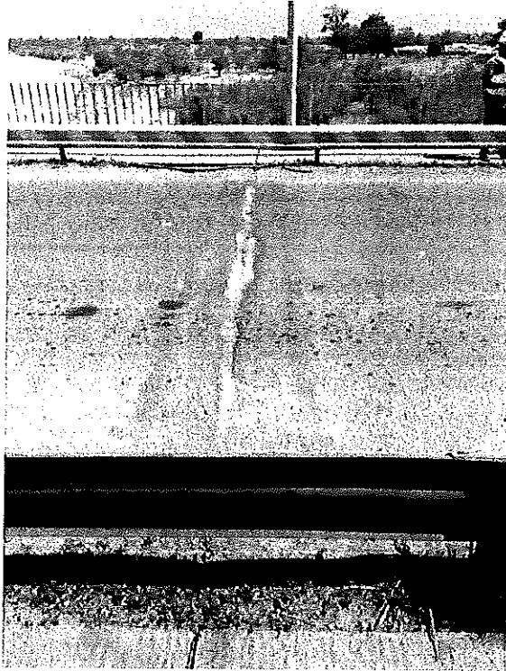
Figure 23. Yapei Bridge. Pavement close to Intermediate joint between slab segments.
